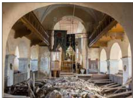
Deckeneinsturz in Alzen
