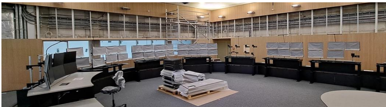
Figure 118: Main Control Room of the FAIR Control Centre, equipped with consoles including integrated screens.
