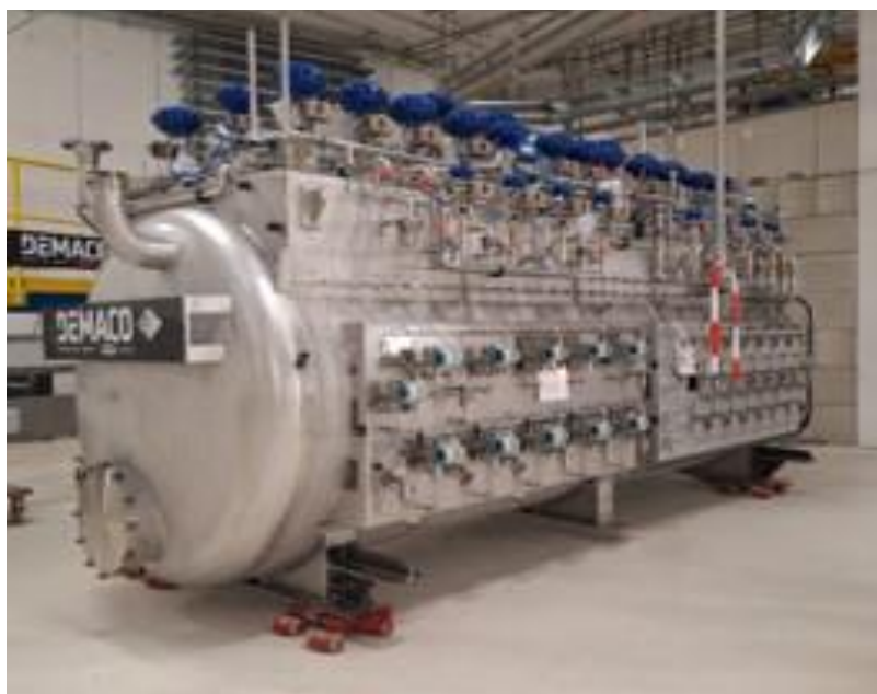
Figure 89: Branch Box, local cryogenics distribution unit.
