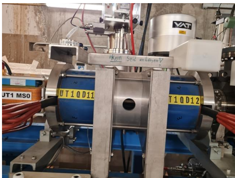
Figure 108: The quadrupole doublet magnet UT1QD11 (UNILAC tunnel the end), to be replaced.
