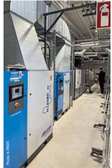
View behind the drying hoppers: Two water-cooled air compressors (in blue at the front) transfer the heat a few metres further to the water heat exchangers of the dry air generators (at the back).
