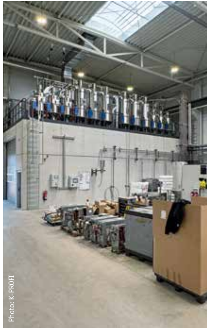
The central material supply with twelve drying hoppers is installed on a concrete platform and is supplied via the outdoor silos or via big bag emptying stations under the platform.
