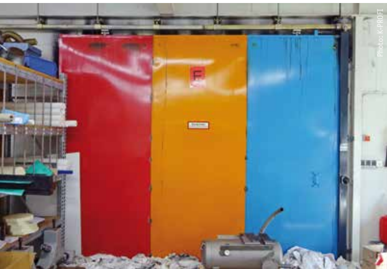
The fire protection doors to neighbouring halls withstood the forces, as did the fire wall to Wefapress' newest warehouse to date.
