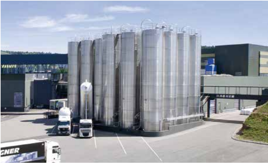
The silos for the incoming PET are located close to the building and are equipped with vibrating floors to avoid clumping of the flakes obtained from bottles.
