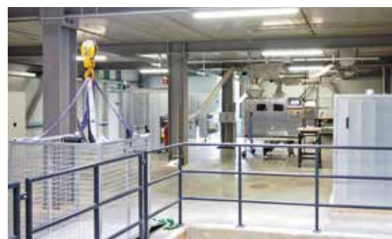
On the level below, the actual sorting takes place in a maximum of four passes on one of the five optical sorting systems.
