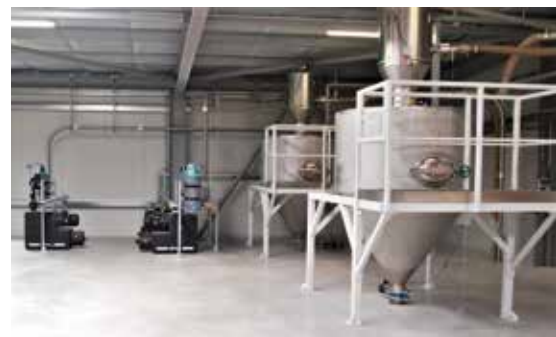
The sorting process begins in the production hall in Niederzissen on the second level with the material feed.
