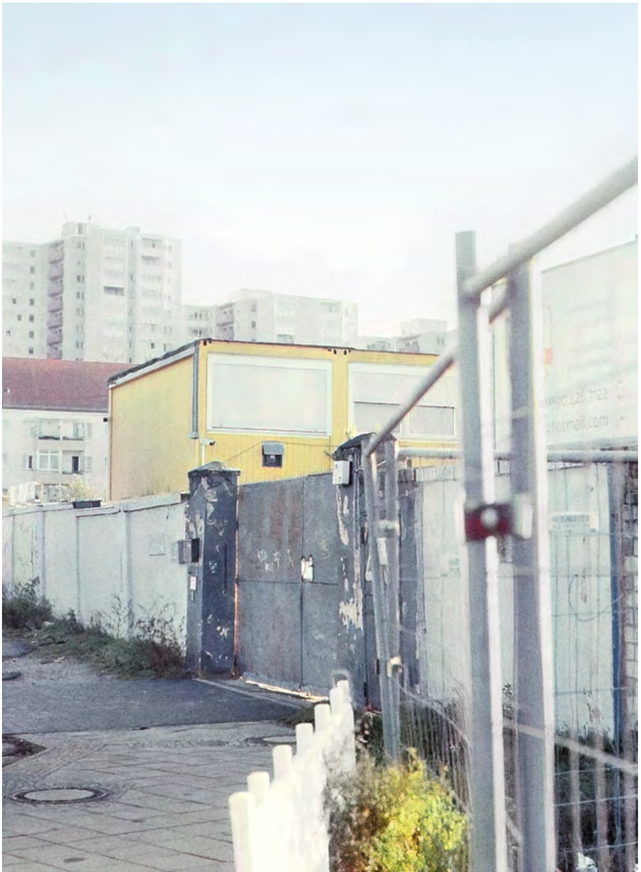
The "white estate" in Berlin-Neukölln is affected by intolerable building conditions, but refurbishment would mean high rent increases. Photo: Firdes Firat
