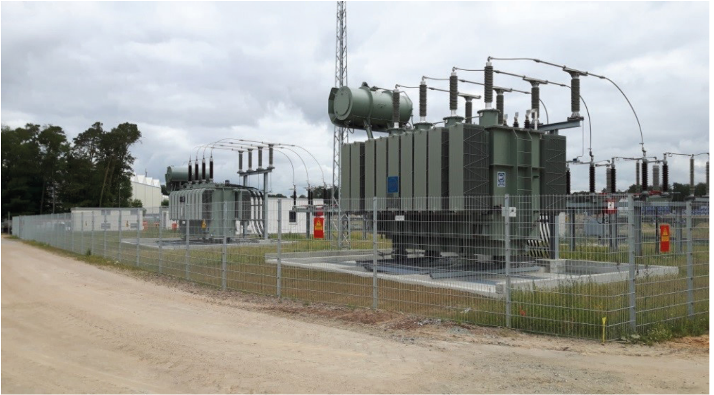
Figure 53. FAIR transformer station south
