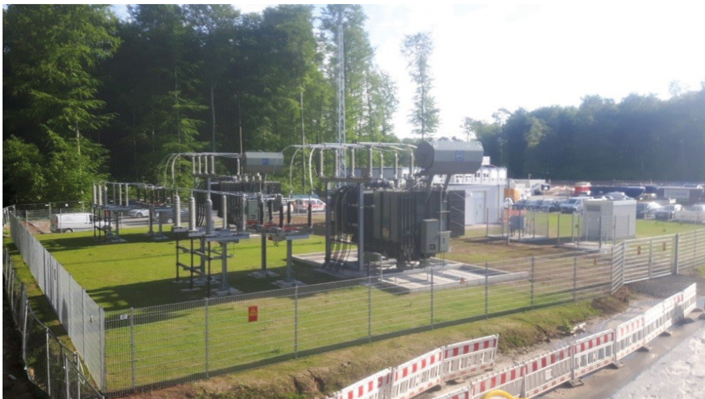
Figure 52. FAIR transformer station north
