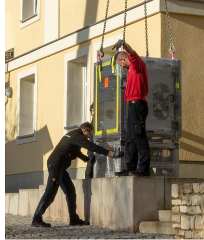
Figure 2: Delivery of one vacuum-module
