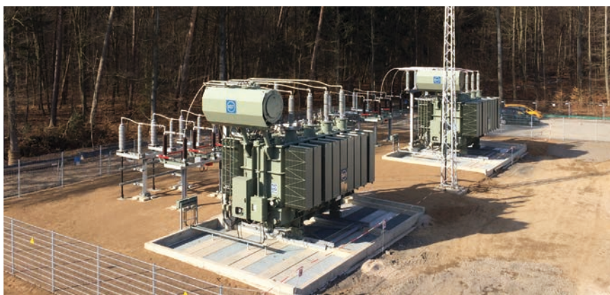
Transformer station North on the FAIR construction site.
