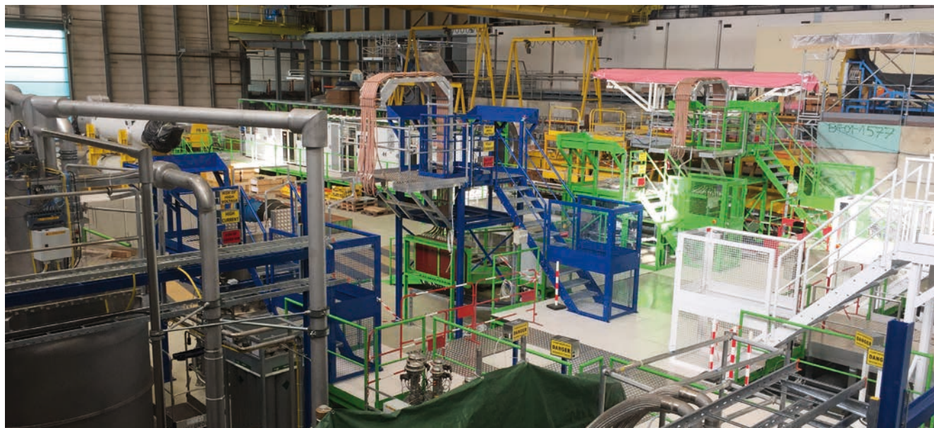
The test facility for magnets at CERN will be used to test multiplets for the Super-FRS.
