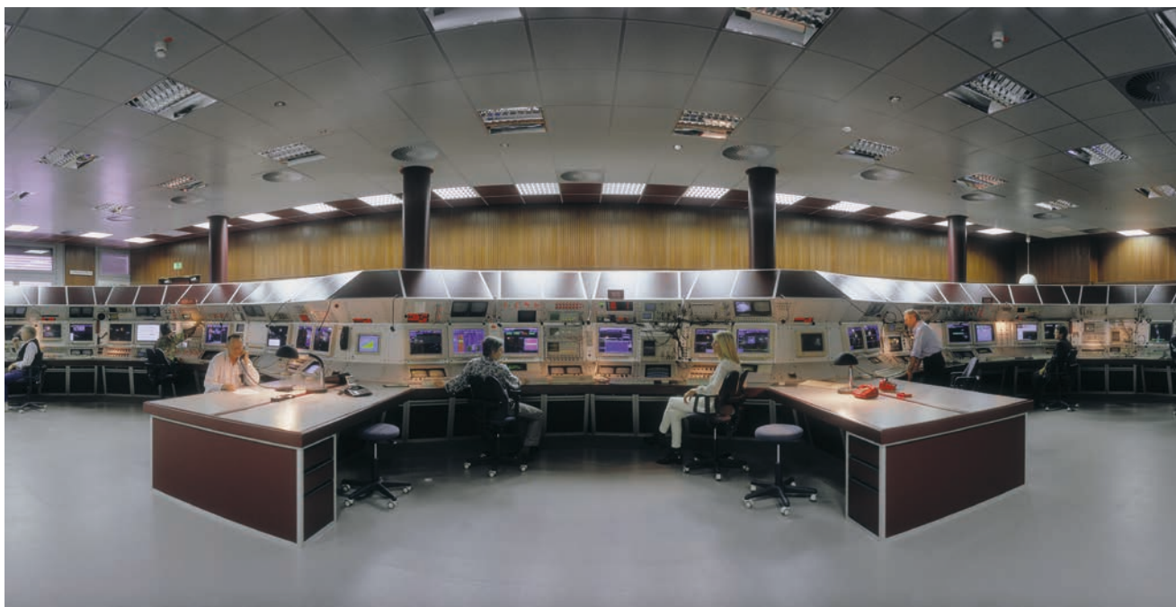
The main control room is the heart of the accelerator facility. The panorama shows the configuration from 1998.
