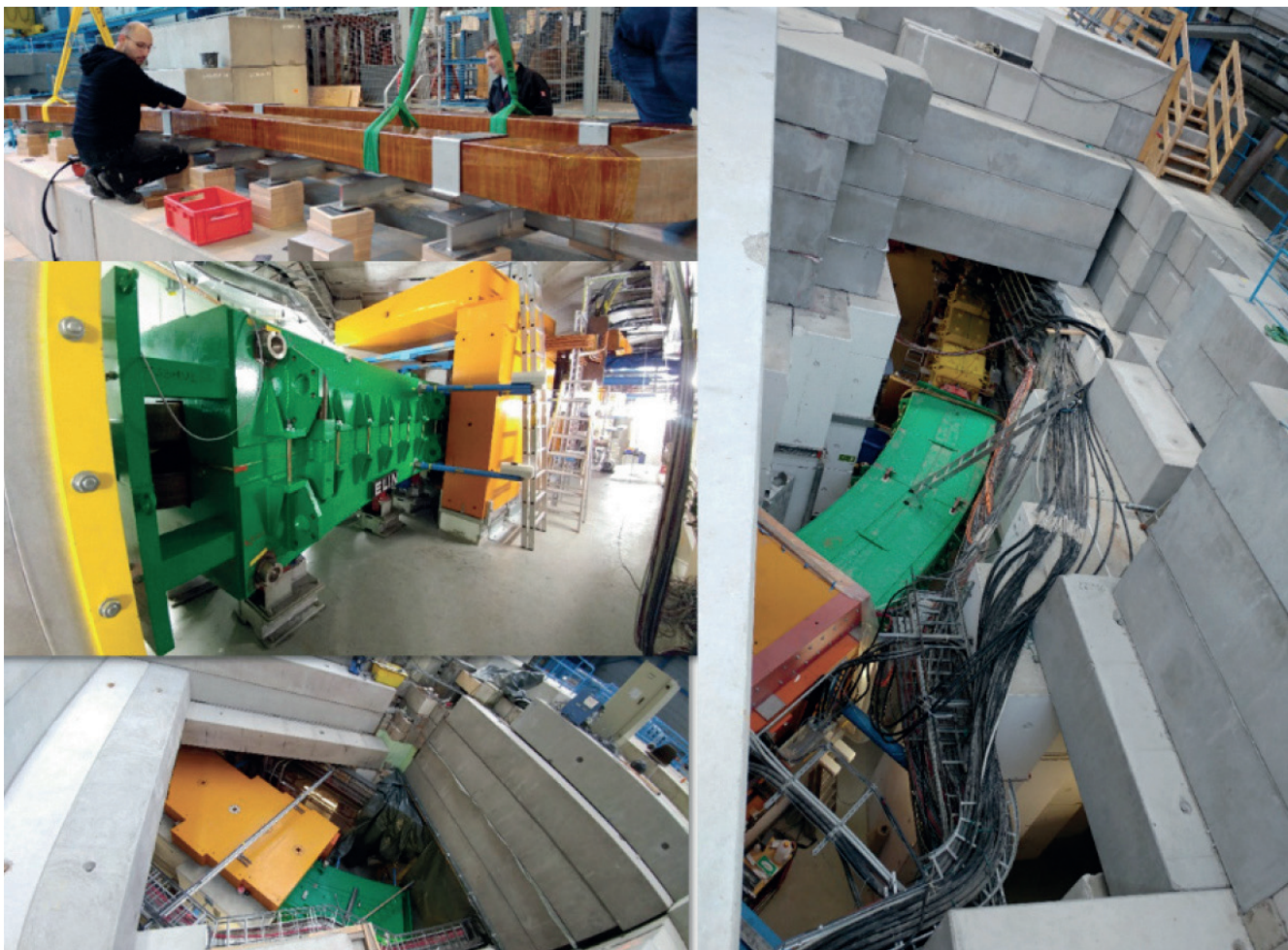
Figure 29. Views into the FRS Top left: Upper Coil and vacuum chamber during repair. Middle and bottom left: target area and the first dipole after the repair without concrete shielding. Right: Second dipole after the repair, but before the reinstallation of the concrete shielding.
