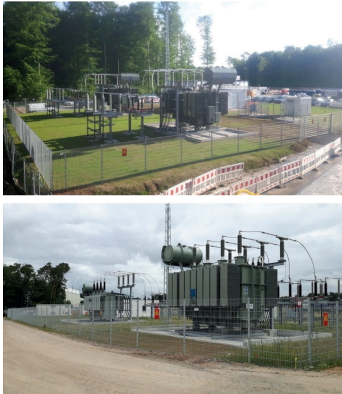
Figure 62. FAIR Transformer Stations North (top) and South (bottom).
