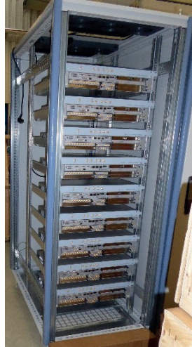
Figure 103. LLRF controllers prepared for SAT.
