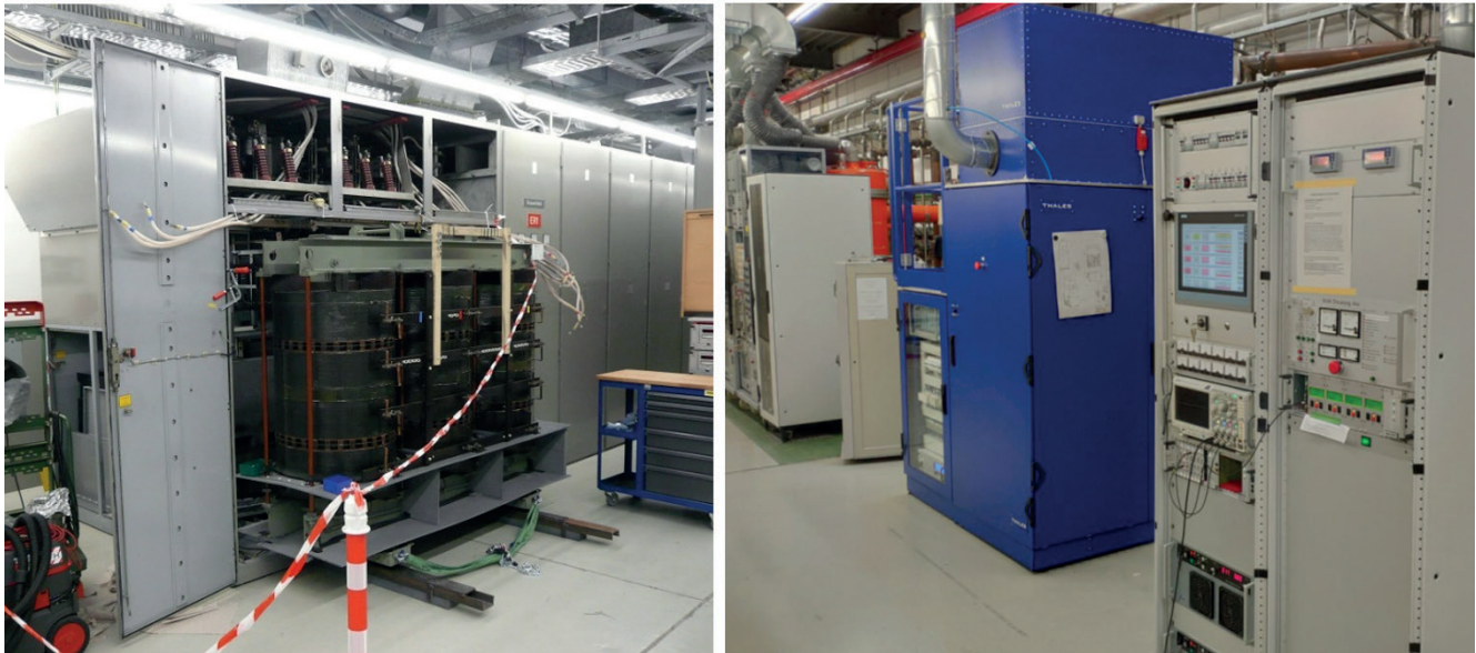
Figure 78. Left: ER1 1 MVA high-voltage power converter with 20 kV transformer (pulled out) during refurbishment. Right: New 1.8 MW Thales high-power RF amplifier and control racks (including PLC, grid power supplies, and further control and interlock components).
