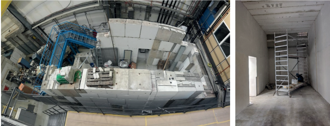
Figure 76. Picture of the new radiation cave for the advanced demonstrator at SH4 during construction (left) and after completion (right).
