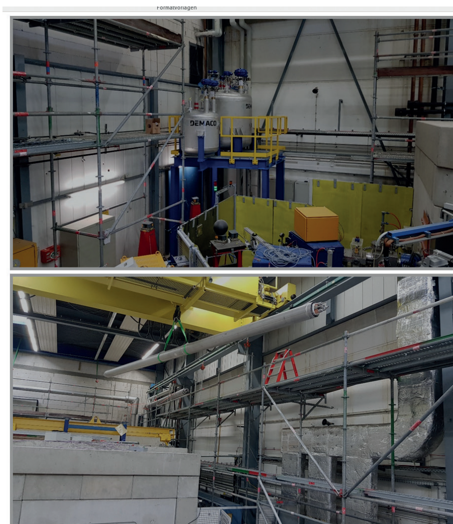
Figure 77. Installation of valve boxes (top) and liquid He transfer line (bottom) by DEMACO at SH4.
