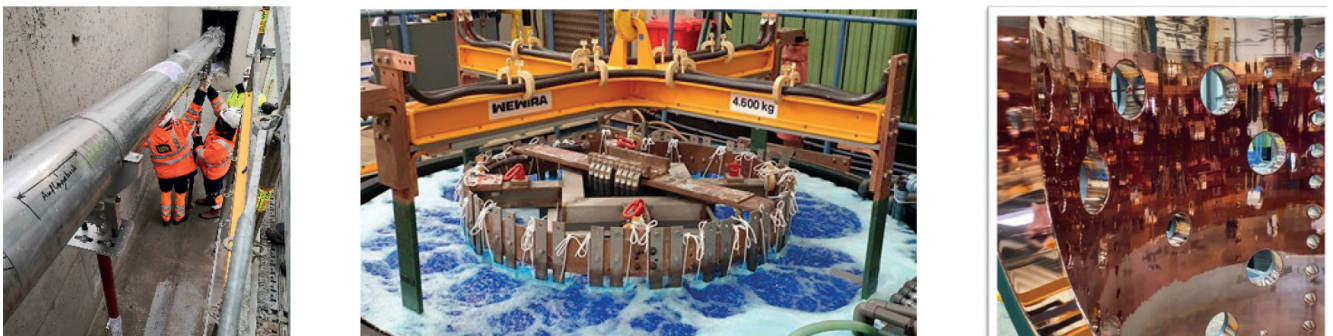
Figure 95. Mounting of the 13 m long Laser beam pipe at FAIR SIS 100 construction site. – mid: Large demo tank for Alvarez tank during Cu plating. – right: The tank directly after Cu plating.
