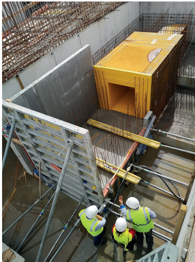
Figure 100. Iron part of the pbar beamdump before it was covered with concrete.
