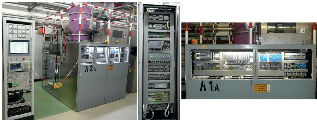
Figure 68. New control cabinet (leftmost) and high-power RF amplifier (HPA) of the ALVAREZ tank A2a after refurbishment (left photo). Backside of one of the new control cabinets (centre) and mounting panel with PLC sub-unit and further electrical equipment at the A1 HPA (right).
