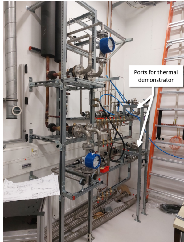
Figure 3: Cooling test rig during assembly.
