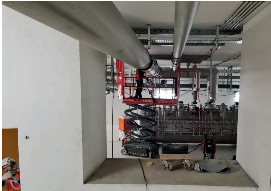
Figure 96. Part of the distribution system in niche 5.
