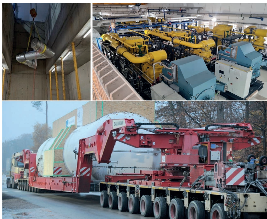
Figure 84. Top left: Cryo 2 installed in Cryo building on site – Top right: Start of component installation on FAIR site – Bottom: Delivery of the Cryo2 Cold Box.
