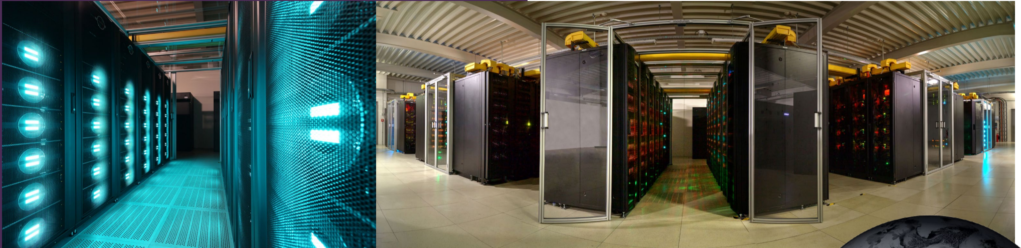
▲ Photo 5.4-2: View into the DKRZ's disk storage system
