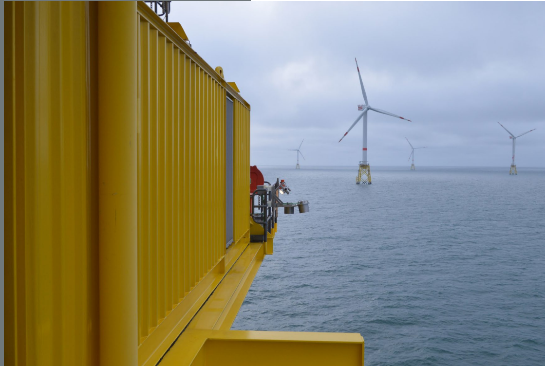
◀ Photo 3.5-2: At half of the measuring stations, redundant measurements are or were carried out using wave buoys or wave radars. In this offshore wind farm, the wave radar is fixed to the substation platform. Redundant measurements serve to compare the different measurement systems and improve data quality control methods.
