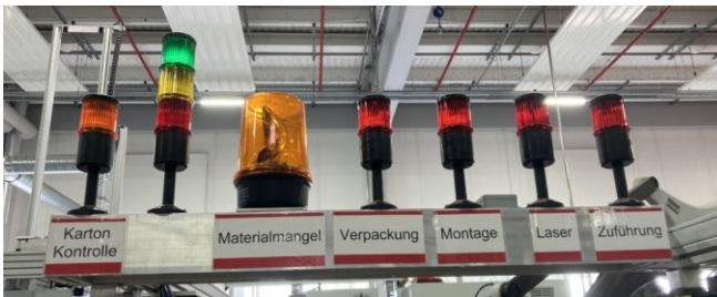
Figure 132: Multiple stack lights from Fischer, text from left packaging check; lack of material (flashing); packaging; assembly; laser; feeder (Image Fischer with permission)
