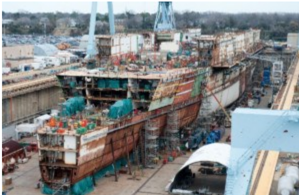
Figure 259: USS Gerald R Ford CVN 78 under construction (Image Ricky Thompson in public domain)
