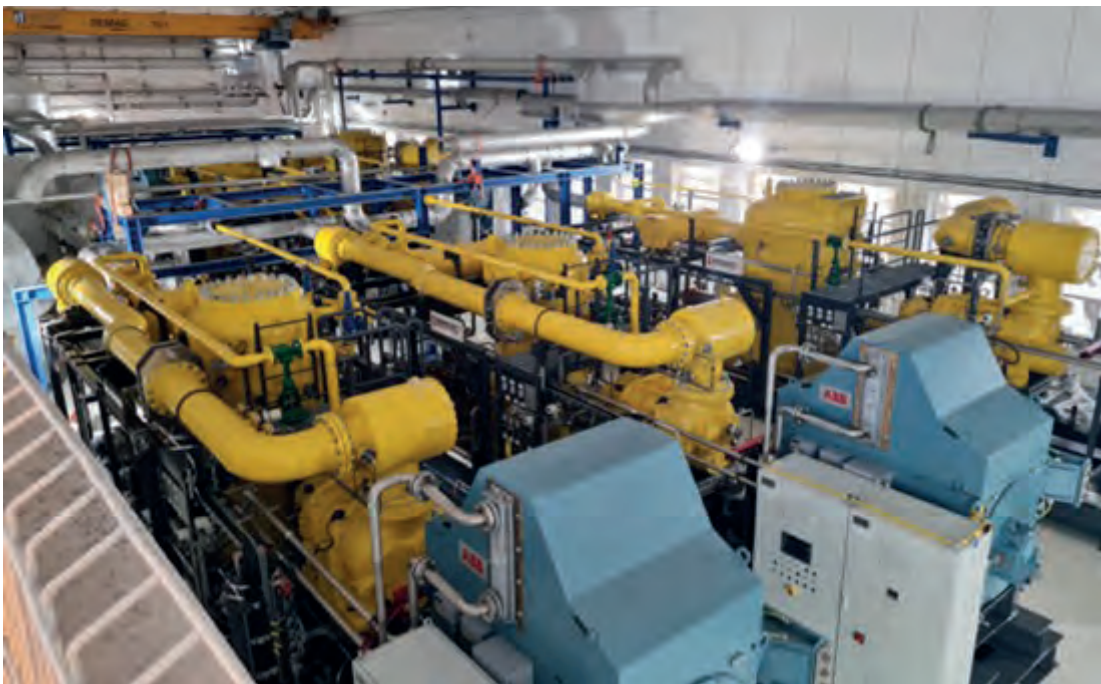
Figure 124. Compressor system for CRYO2 and CWU
