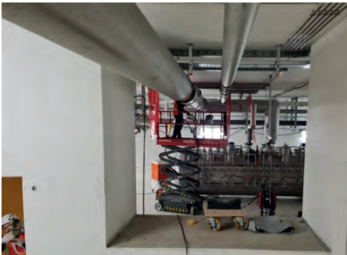
Figure 125. Part of the distribution system in niche 5
