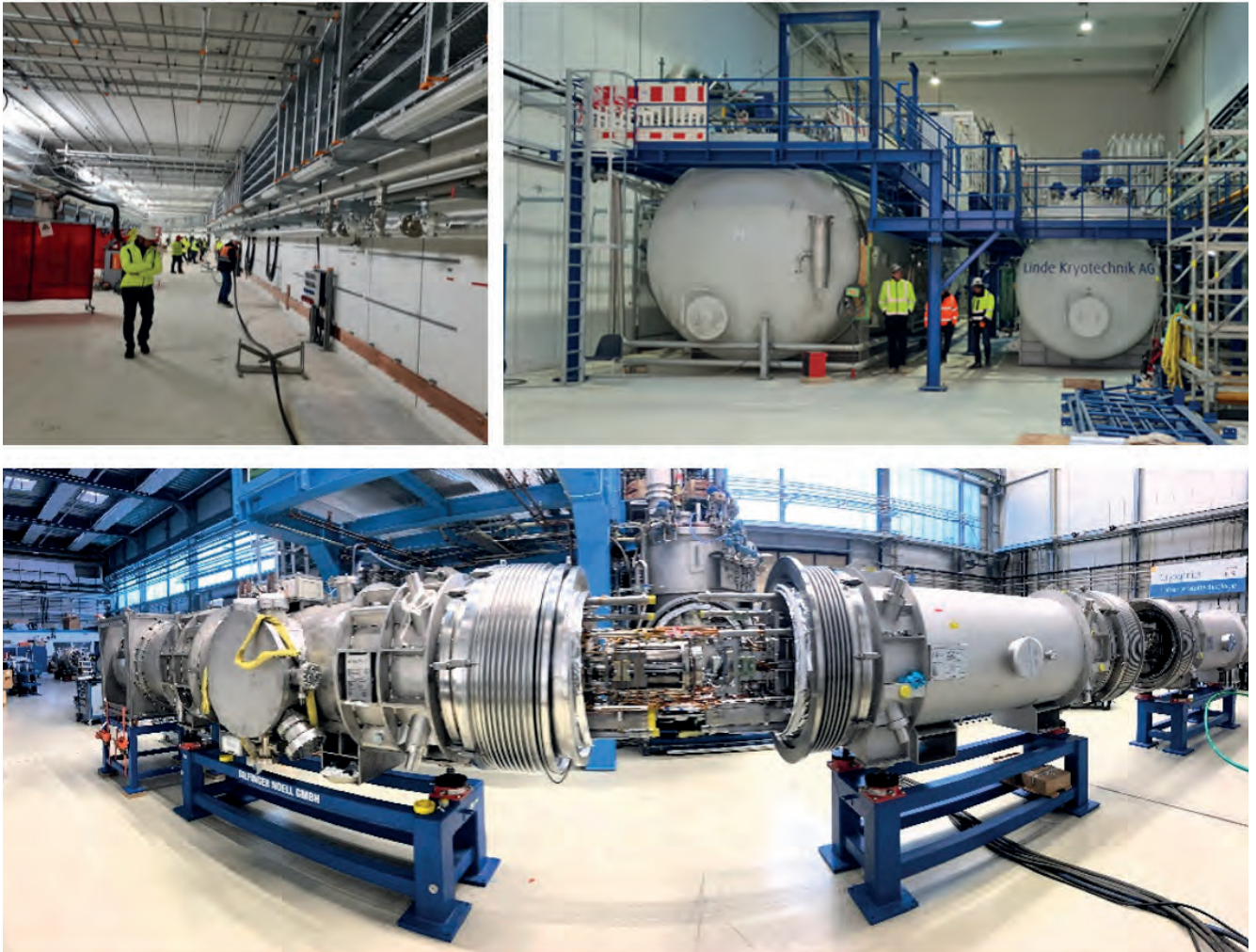
Figure 114. Top left: Start of cable pulling in the SIS100 tunnel – Top right: Cryo Plant installation completed – Bottom: SIS100 string test
