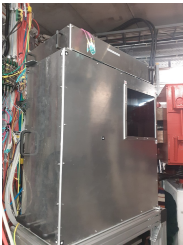
Figure 5: Service box for the new mSTS module on top of the existing mSTS box.
