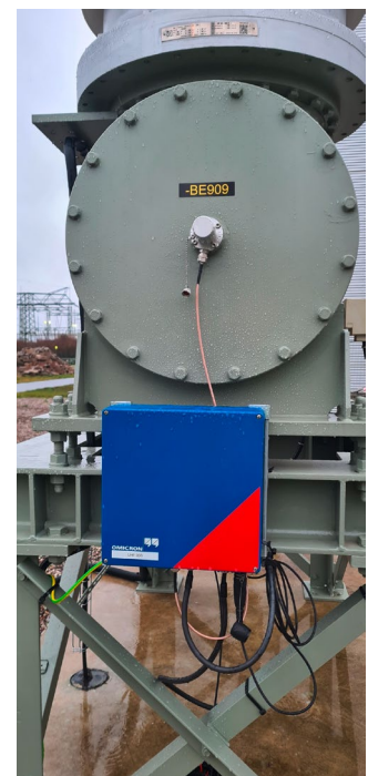
Fig. 6: Long duration measurement system installed at the GIS
