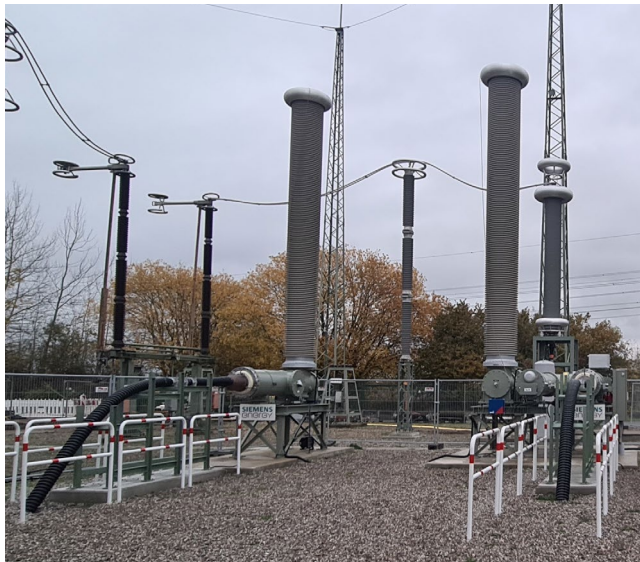
Fig. 1: Successfully installed HVDC GIS in Bentwisch
