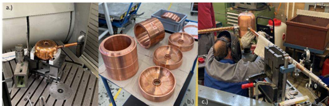
Figure 89: Drift tubes for existing Alvarez at UNILAC. Part a.) shows the repair of a leakage of the inner cooling pipe of a drift tube by means of soldering. b.) shows newly manufactured parts of a drift tube for Alvarez A I. The right panel c.) shows the welding of the stems of the A I drift tube.
