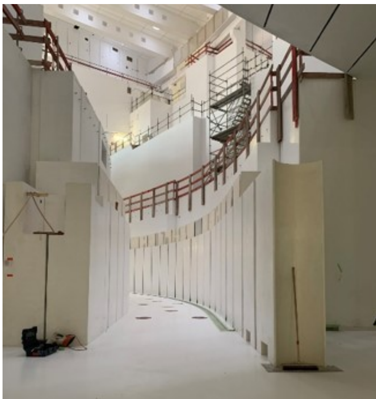
Figure 70: View of the narrow iron shielding tunnel of Super-FRS target area.
