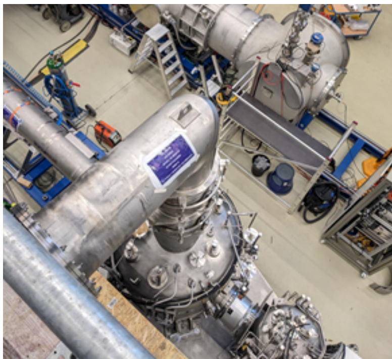
Figure 77: Super-FRS local cryogenic assembly of transfer line, feed box, end box and jumper connection to the magnet, installed at the STF
