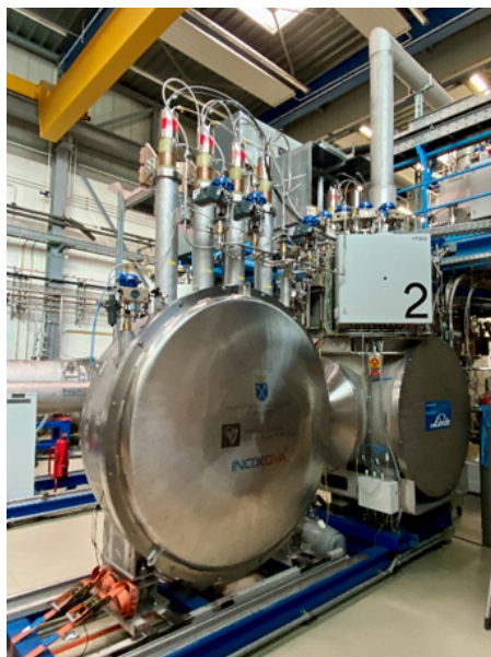
Figure 69: The FOS current lead box at cold testing at the GSI series test facility (STF)
