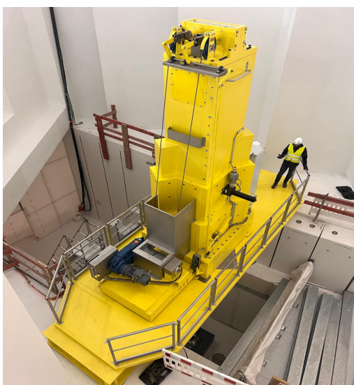
Figure 62: Super-FRS Flask delivered and installed on site
