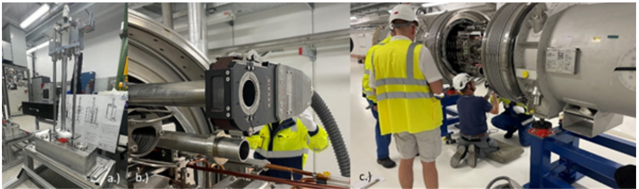
Figure 91: Support of the FAIR project. a.) shows the drive units for Super-FRS, b.) show the orbital welding gun test placement, and c.) shows preparative work for the welding connections on SIS100 dipoles.
