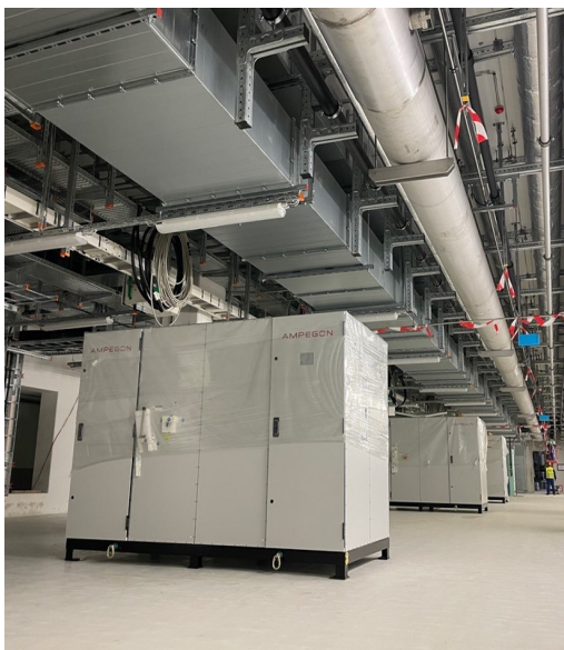
Figure 61: First Power Supply Unit in the SIS100 tunnel
