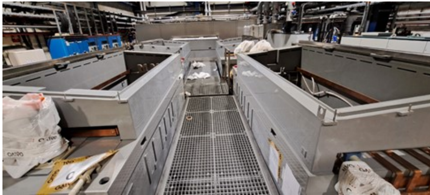
Figure 100: Cu plating line for the drift tubes during set up @ CERN (L. Ferreira, CERN)
