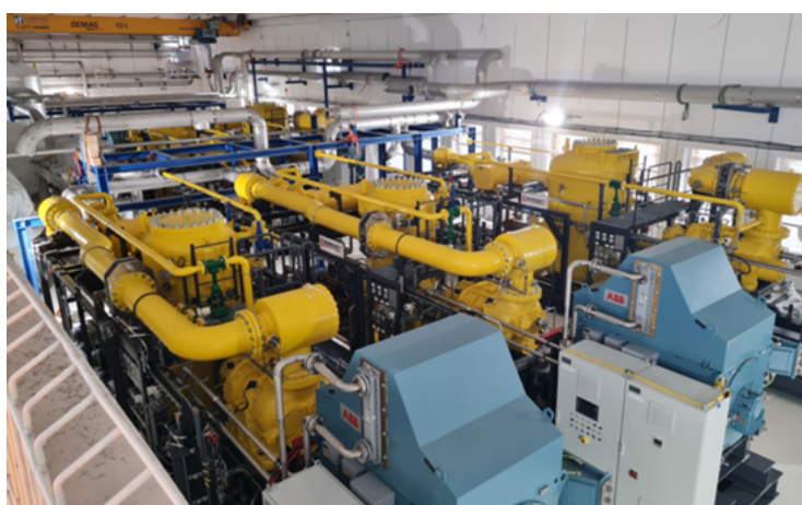
Figure 79: Compressor system for CRYO2 and CW
