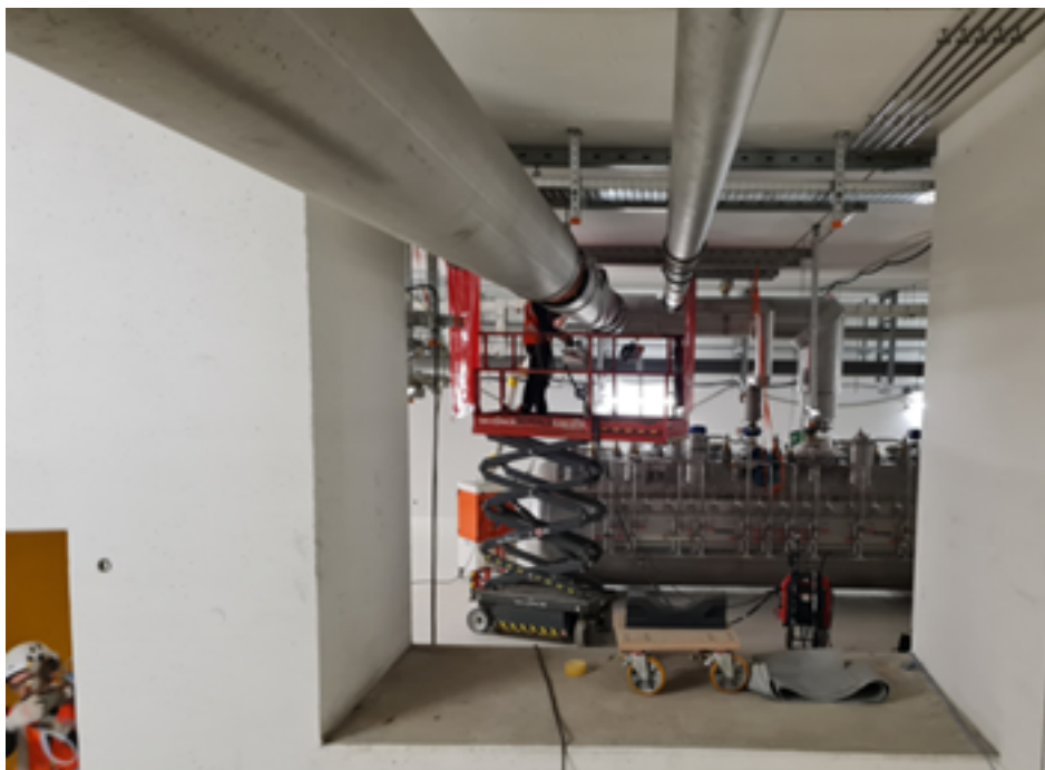
Figure 81: Part of the distribution system in niche 5
